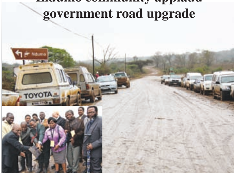
KwaZulu-Natal MEC for Transport, Community Safety and Liaison Willies Mchunu and Head Of Department Chris Hlabisa sod turn the gravel road P435 in Indumo near Jozini.
